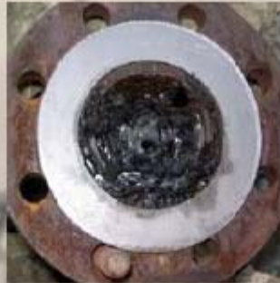
Diaphragm is corroded
